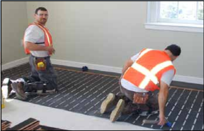
District Council 16 Members working in San Francisco at the Presidio Landmark Project.
